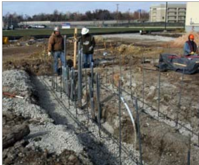
Apache Corp. is constructing a CNG filling station at 5011 S. Vandalia Ave. in Tulsa. (Rip Stell)
