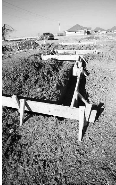
The early stage of a new home under way by Jeff Click Homes is shown at 2120 NW 172 in March. Click is among those building smaller houses in response to increased demand. This home has 1,398 square feet.
