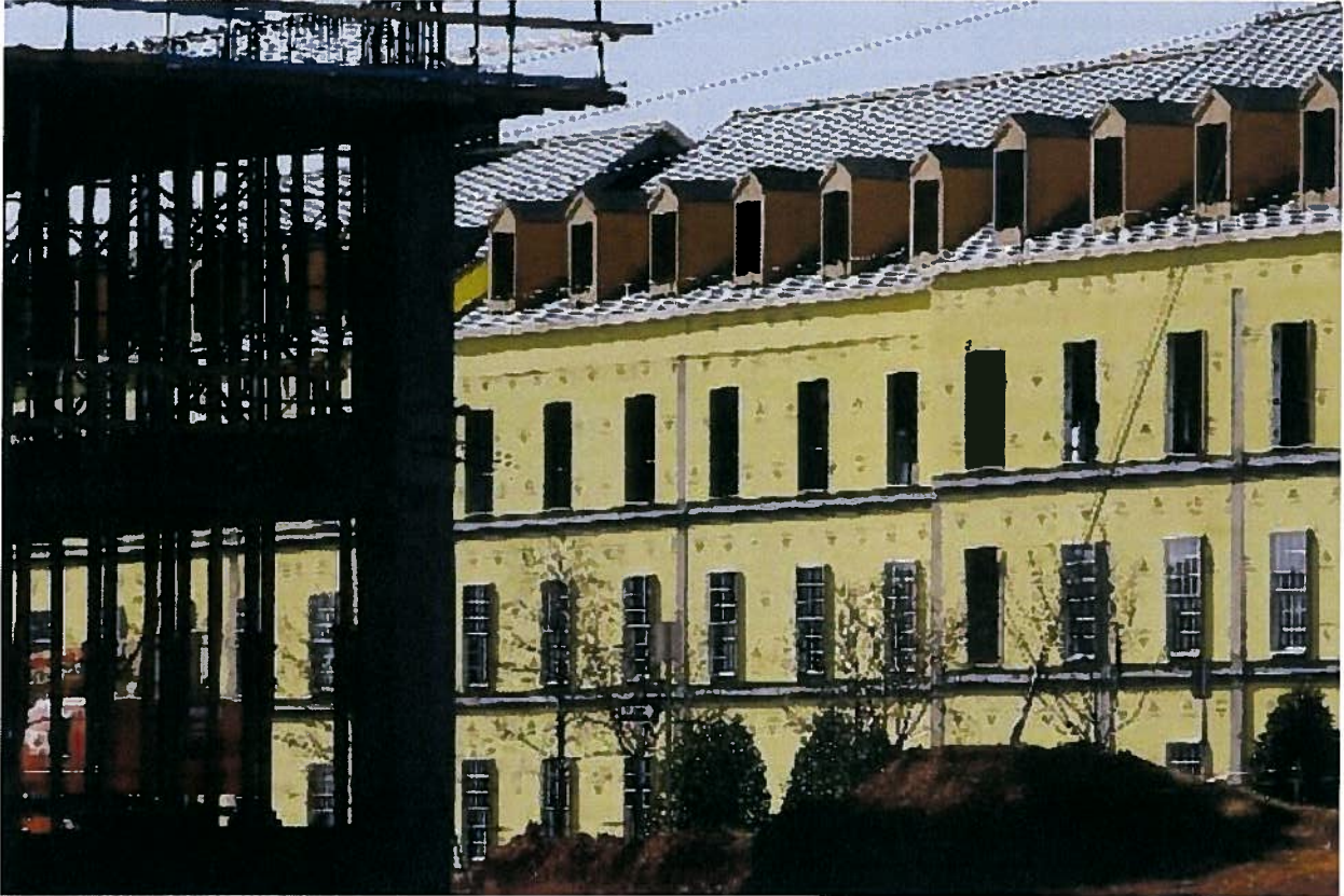
Ongoing construction on the campus of Chesapeake Energy near NW 63 and Classen Friday, Jan. 9, 2009. BY JIM BECKEL,
