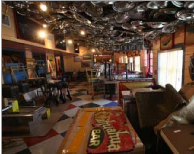
Chuy's Restaurant under construction at 10808 E. 71st St. in Tulsa. (Photos by Rip Stell)
