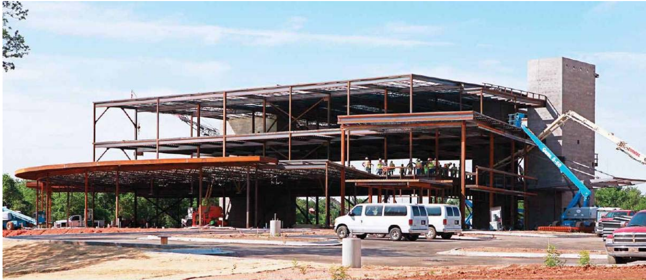
St. Anthony Healthplex South is under construction southeast of Interstate 44 and SW 134. The three-story 52,000-square-foot building is a twin, with the other one under way at Interstate 40 and Douglas Boulevard in Midwest City.
