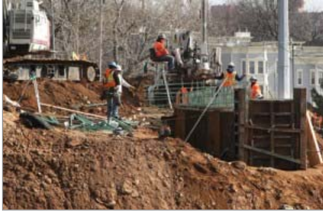
Workers prepare to pour a bridge pier on the I-244 Arkansas River overpass near downtown Tulsa. (Rip Stell)
