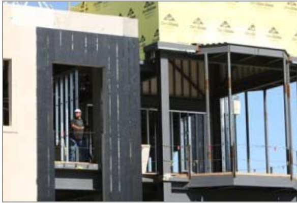
Workers ready Stephenson Hall for installation of its windows. The new hall on the University of Tulsa campus will house the petroleum and mechanical engineering programs. (Rip Stell)
