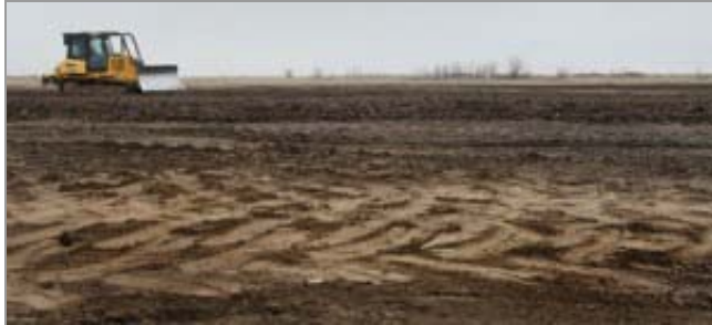
American Tire Distributors hopes to start actual construction in March on its planned center, with a finishing date in July. (Rip Stell)
